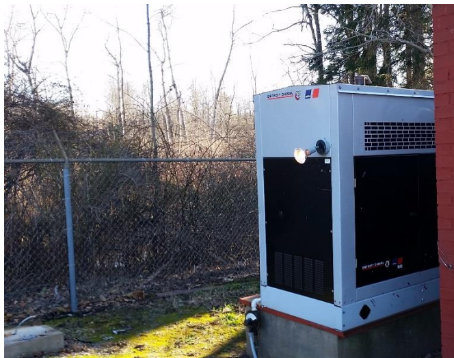
Photo 2-2: Well Site Generator
