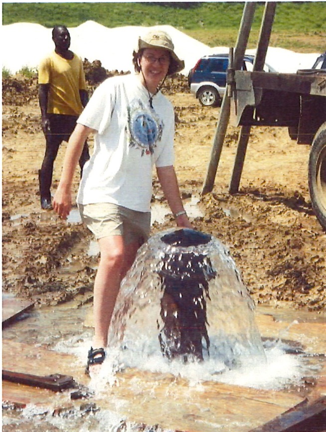
HSA-sited and developed well exhibiting >450 gpm of natural artesian flow that has now continued unabated for over 15 years.
